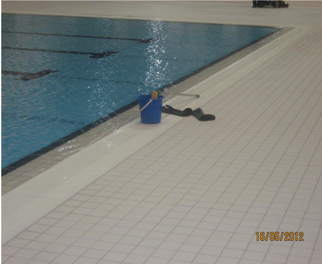
2012 – even new pools can require interventions
