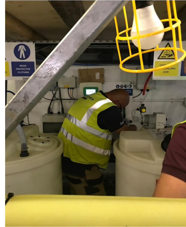
The plant room for the temporary training pool
